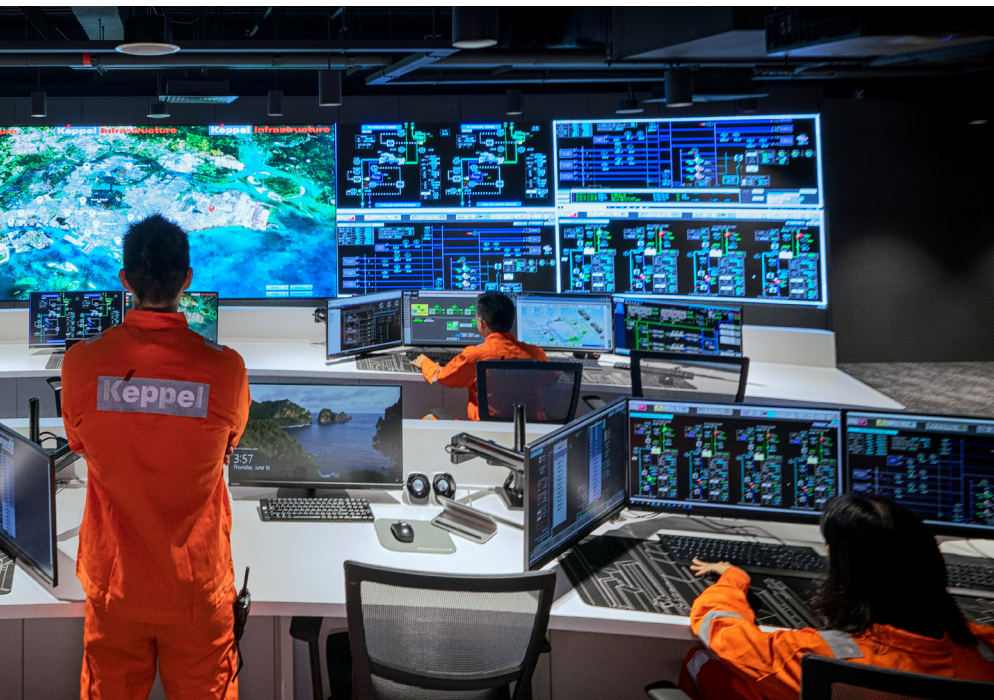
Figure 1 Keppel's state-of-the-art Operations Nerve Centre (ONC)
