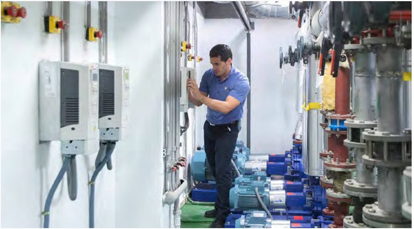
Figure 3 – ABB VSDs and motors have helped the InterContinental hotel in Madrid cut its energy bills by 40%.
